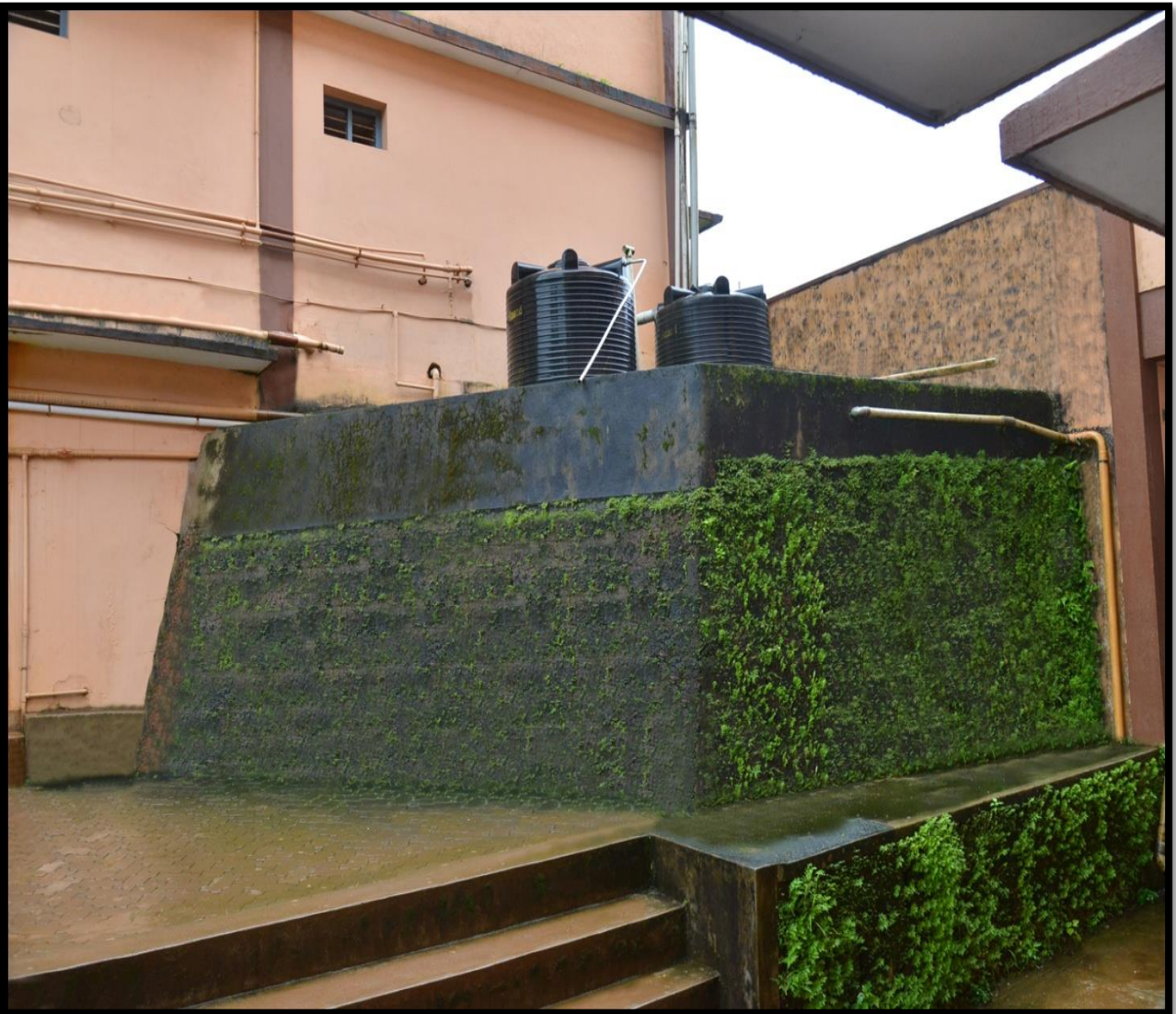
Water Collection Tank
